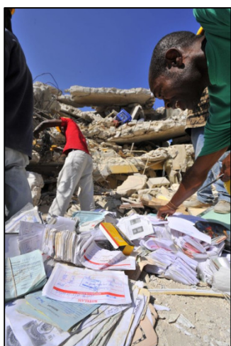
Credit union workers retrieve forms from the crumbled remains of KOTELAM's Magoire Ambrose branch office. Photo by Christian Kober
